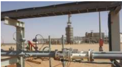
Figure 1. Dynamic liquid metering system of (source: GTFT-Algeria)
